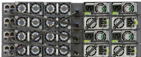
Rear View (highlighting Stackable Chassis cabling)
